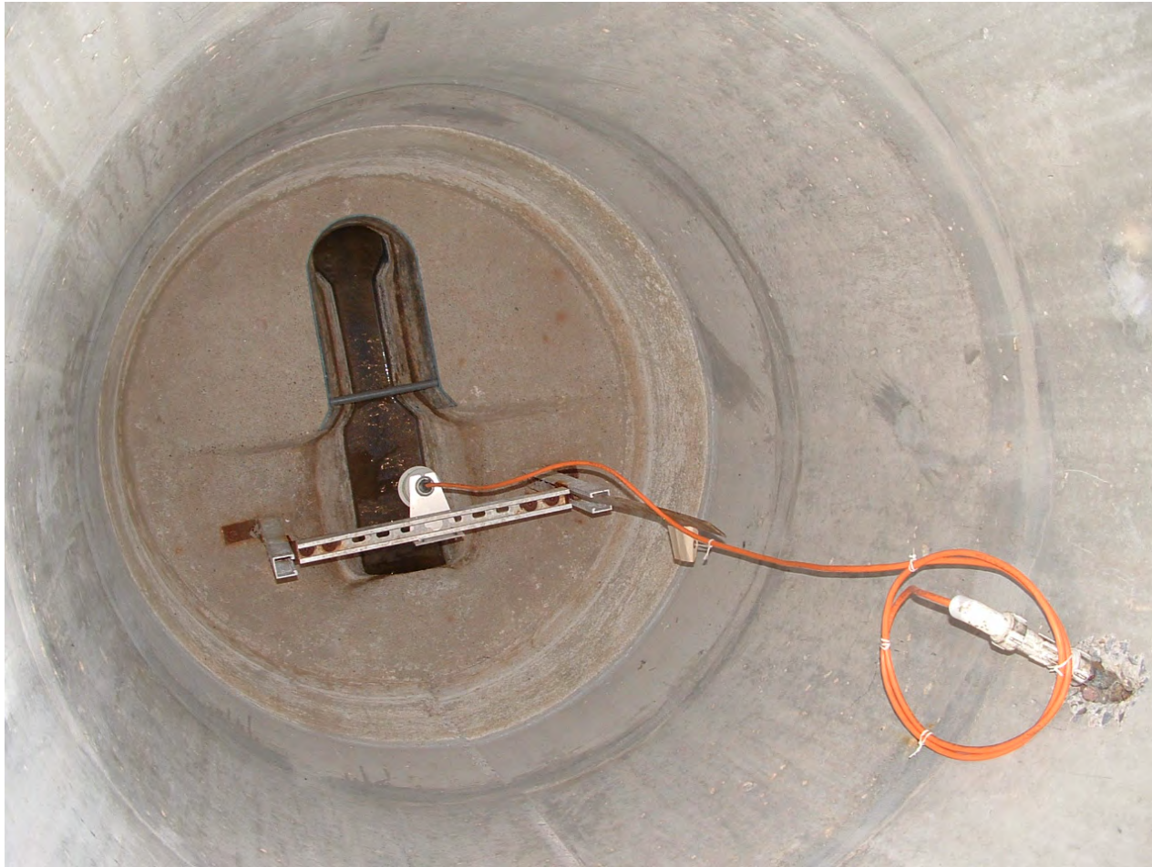
Parchal Flume Flow meter sensor
